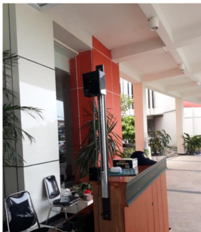
Figure 7 Complete view of temperature detection system
